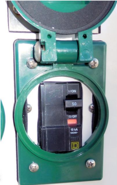
GFI Breaker Roche Harbor
