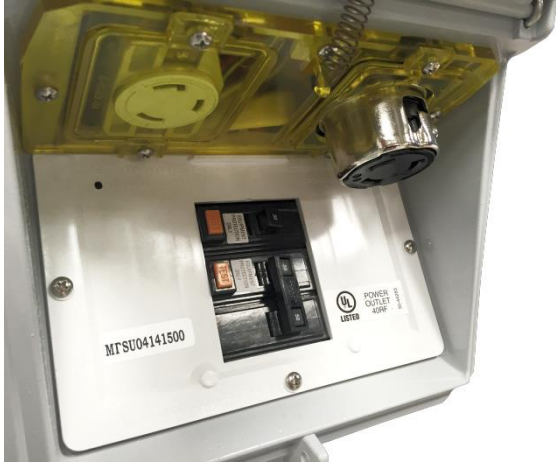
GFI Breaker in an Eaton Lighthouse Pedestal
