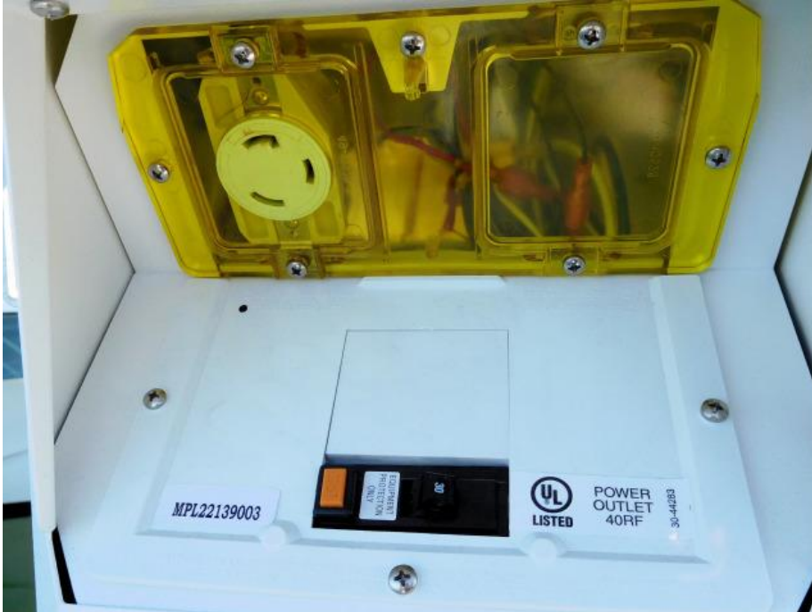
GFI Breaker Eaton Power
